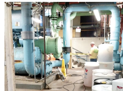
Interior work area showing access difficulties
