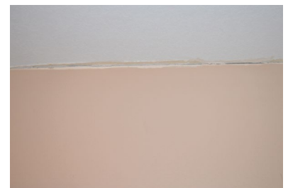
PolyLevel lifted the duplex slab to within 1/8" of its original elevation which dramatically reduced the gap between the ceiling and walls
