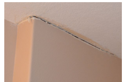
Slab settlement caused visible gaps between partition walls and the ceiling
