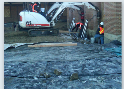
Insulation blankets to prevent further frost penetration
