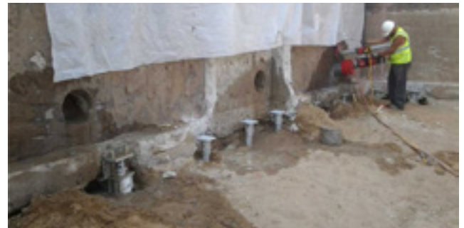
Concrete coring for helical tieback locations above new construction and retrofit helical piles
