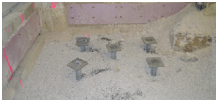
New construction caps welded to installed piles to be cast in new equipment footings
