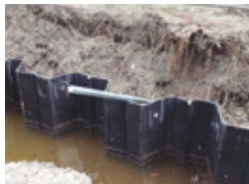
Tieback installed, ready to be cut and fitted with standard new construction bracket
