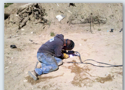
Piles cut to design elevation and new construction brackets tack-welded in place
