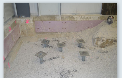
New construction caps welded to installed piles to be cast in new equipment footings
