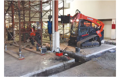
Limited interior access and working space
