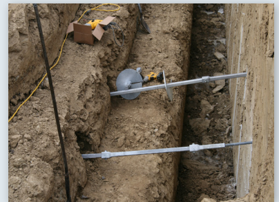
Leads and extensions with helix plates set in place on south side of wall
