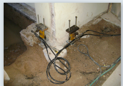
Piers connected in series and uniformly reloaded to the design working load
